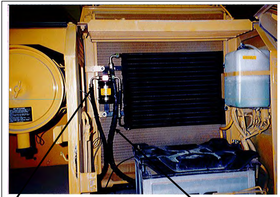
5/16" hose to expansion valve
